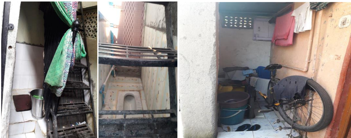
Picture 1: During the SBM toilet survey of Pune Slum in Yerwada Ward “Jyotiba Phule Vasahat” which are incomplete and improperly built up and not have drainage line in December 2017
